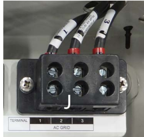
Figure 3-18: Bottom switch AC grid terminal
